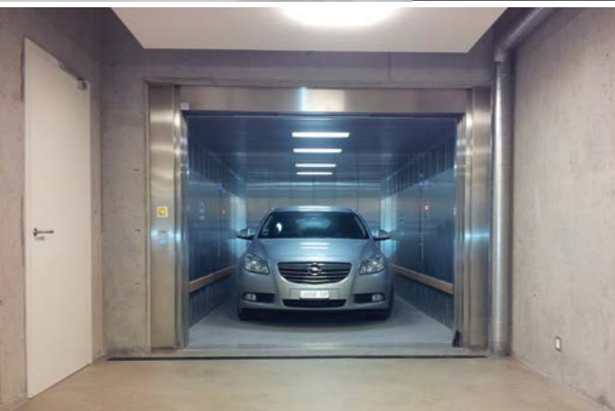
TRAFFICO® Parking, Zürich, Switzerland
