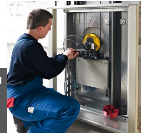
Car lift, Maintenance
